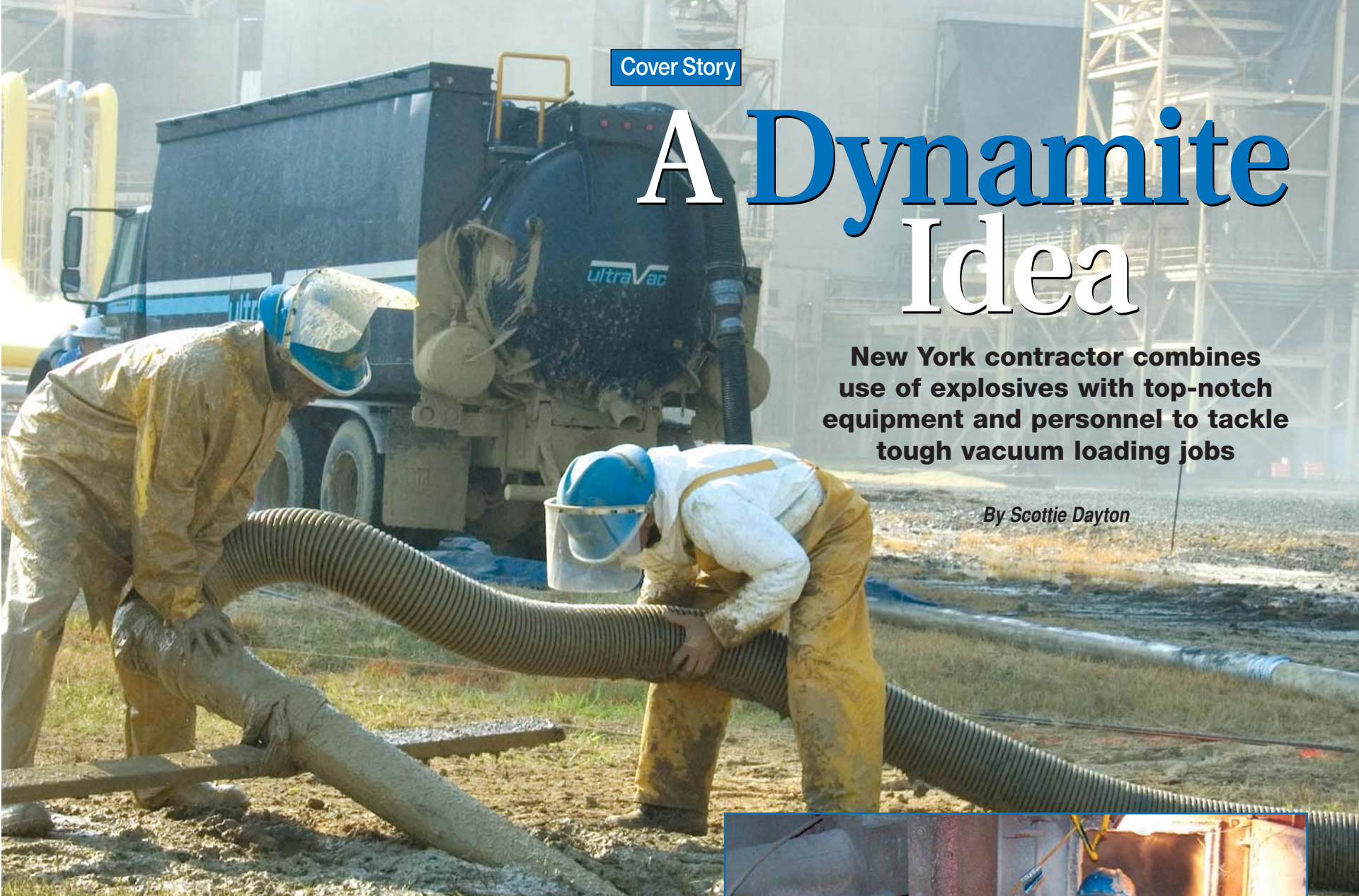
Marcel McCaffity (left) and Danny Alley of North American Industrial Services move a vacuum hose with safety "T" break-off into position at the Chalk Point Generating Plant in Aquasco, Md. (Photos by Val Nyce and North American Industrial Services)
